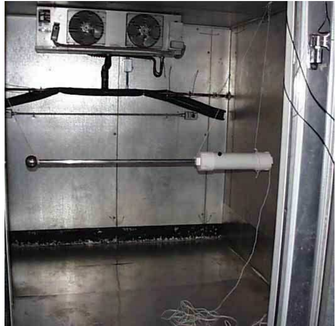
Fig. 9. Experimental test of de-icing a 1 m line. The suspended bar, 1 m long and 25.4 mm in diameter, was coated with 7 mm of ice for the test. The large-diameter white cylinder on the right contains the resonant inductors submerged in oil.
